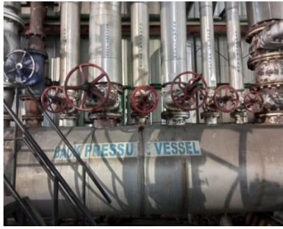
Gambar 4. Back Pressure Vessel di pabrik kelapa sawit
